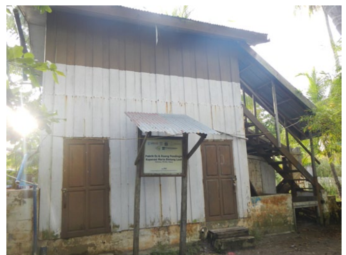
Fig. 6.5: What to do with the disused ice-making facility at Kokonao? A decision-tree can help find the answer.
